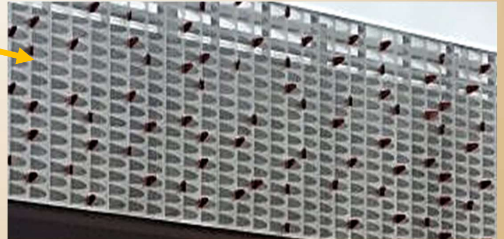
Western Highway upgrade The design included perforated aluminium cladding with red brackets to simulate butterflies.
